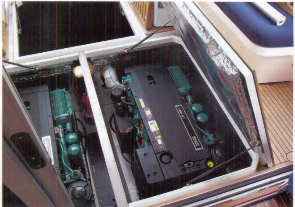
There's plenty of space around the twin Volvos, situated in a large engine room beneath the cockpit sole
